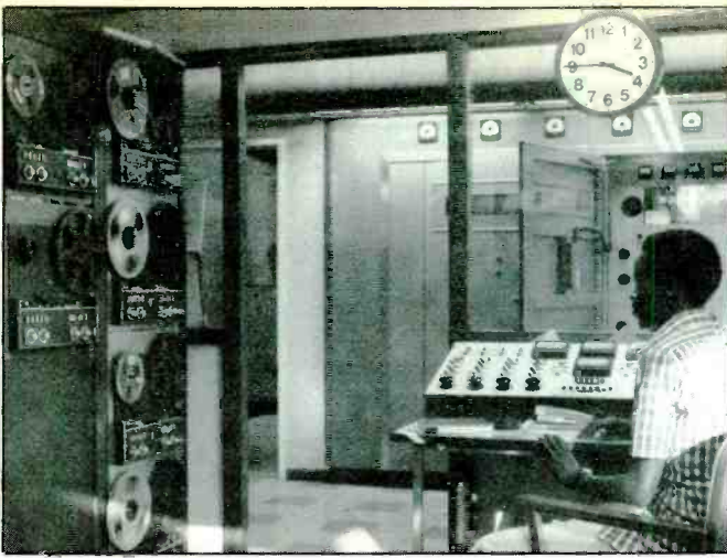
TWR Swaziland. A view of control board and taped programs being fed to transmitters across the hall.
